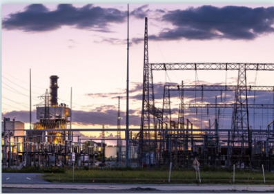
power & distribution Energy Sector
