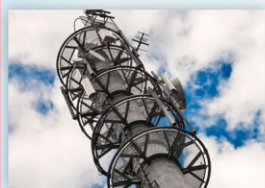
Guyed Mast Towers
