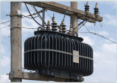
Pole Mounted Transformer
