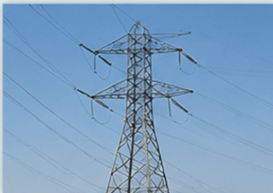
Transmission and Telecom Towers
