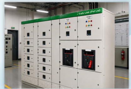
Low Voltage Switchgear
