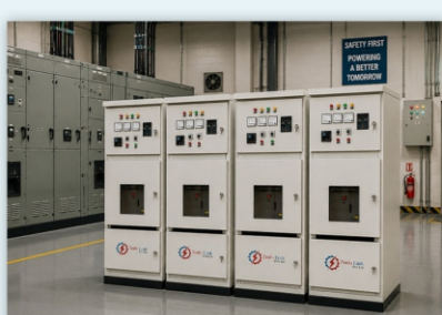
Medium Voltage Switchgear
